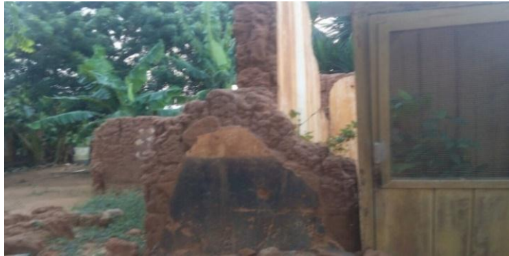
Plate2: Collapsed building at Klo-Begro
