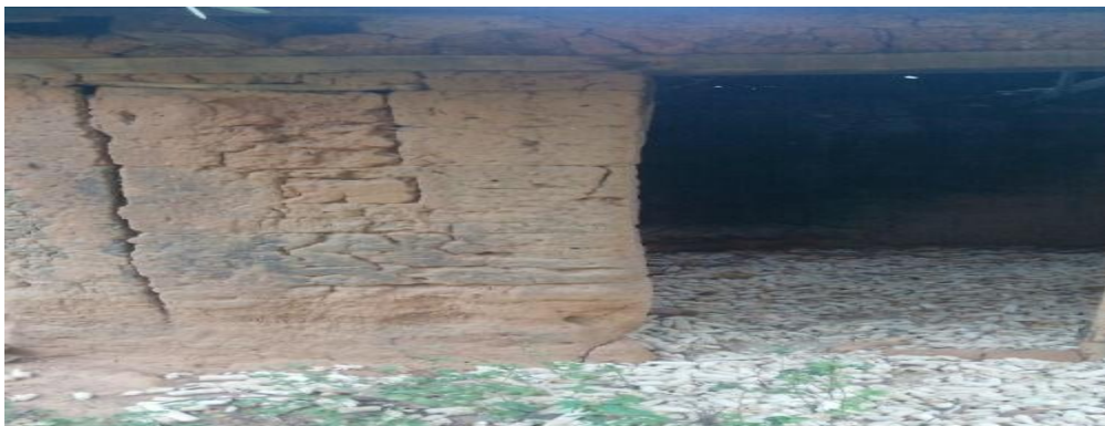
Plate 1: Cracked building at Odugblase
